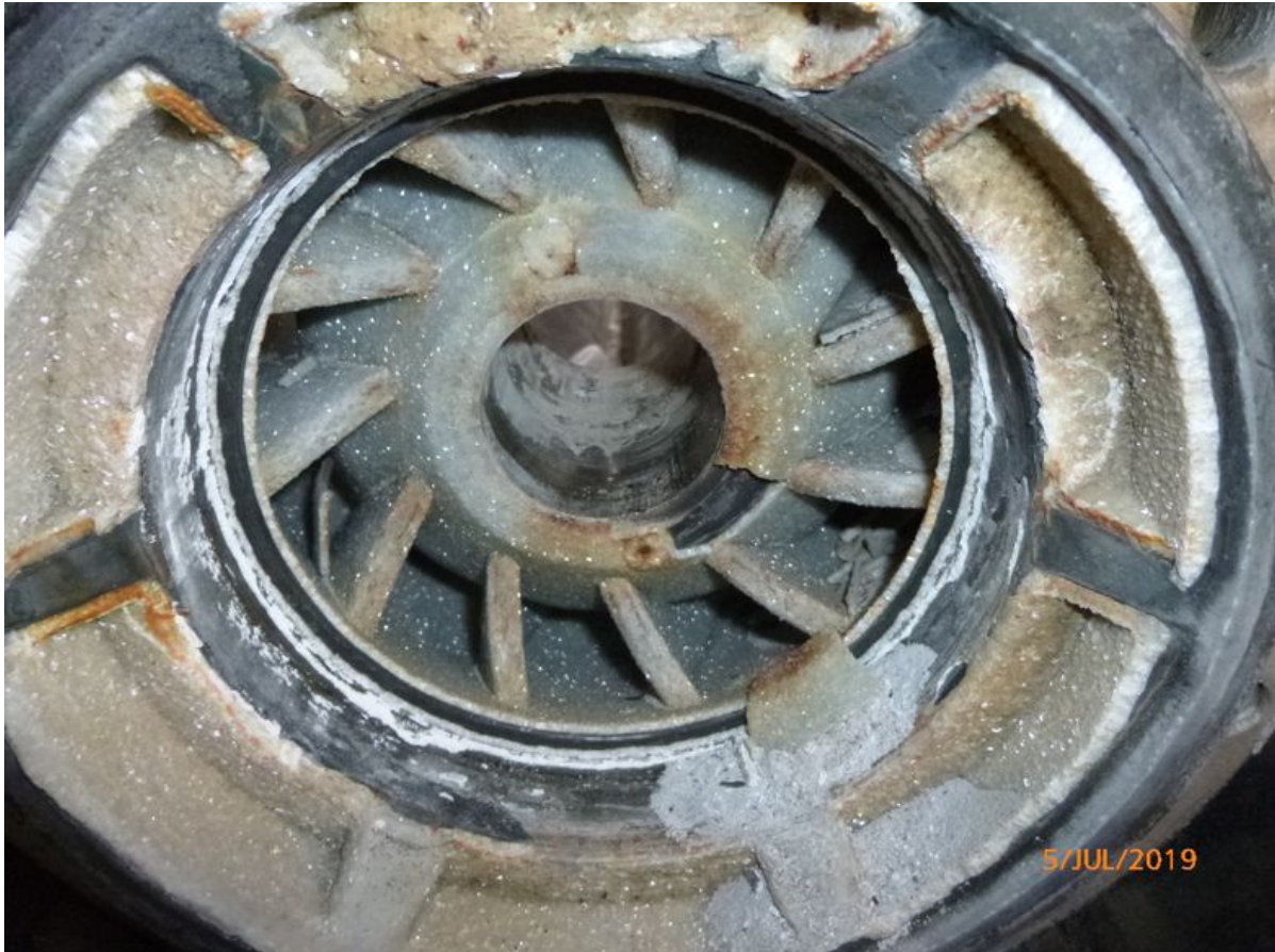
A pump stage with typical lime deposits
