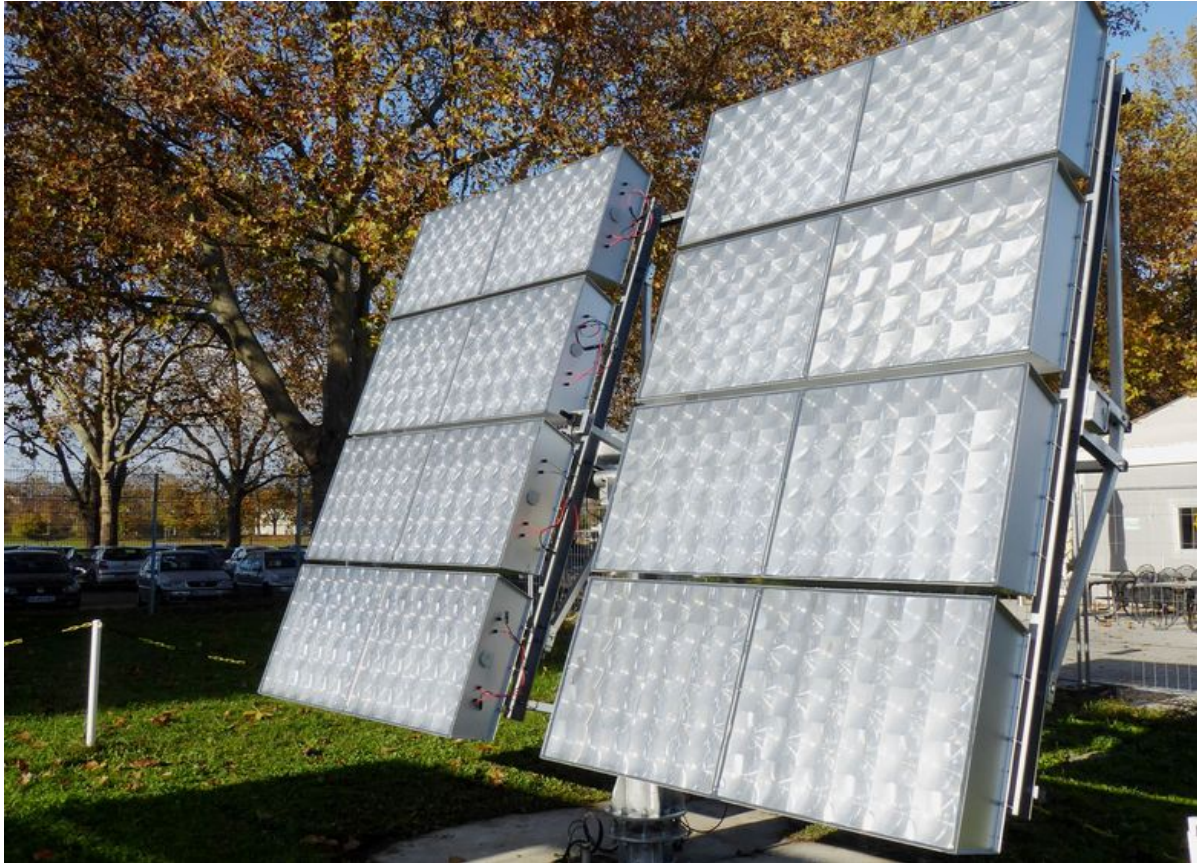
Concentrator photovoltaic modules fully installed on a dual-axis tracker in Heilbronn.
